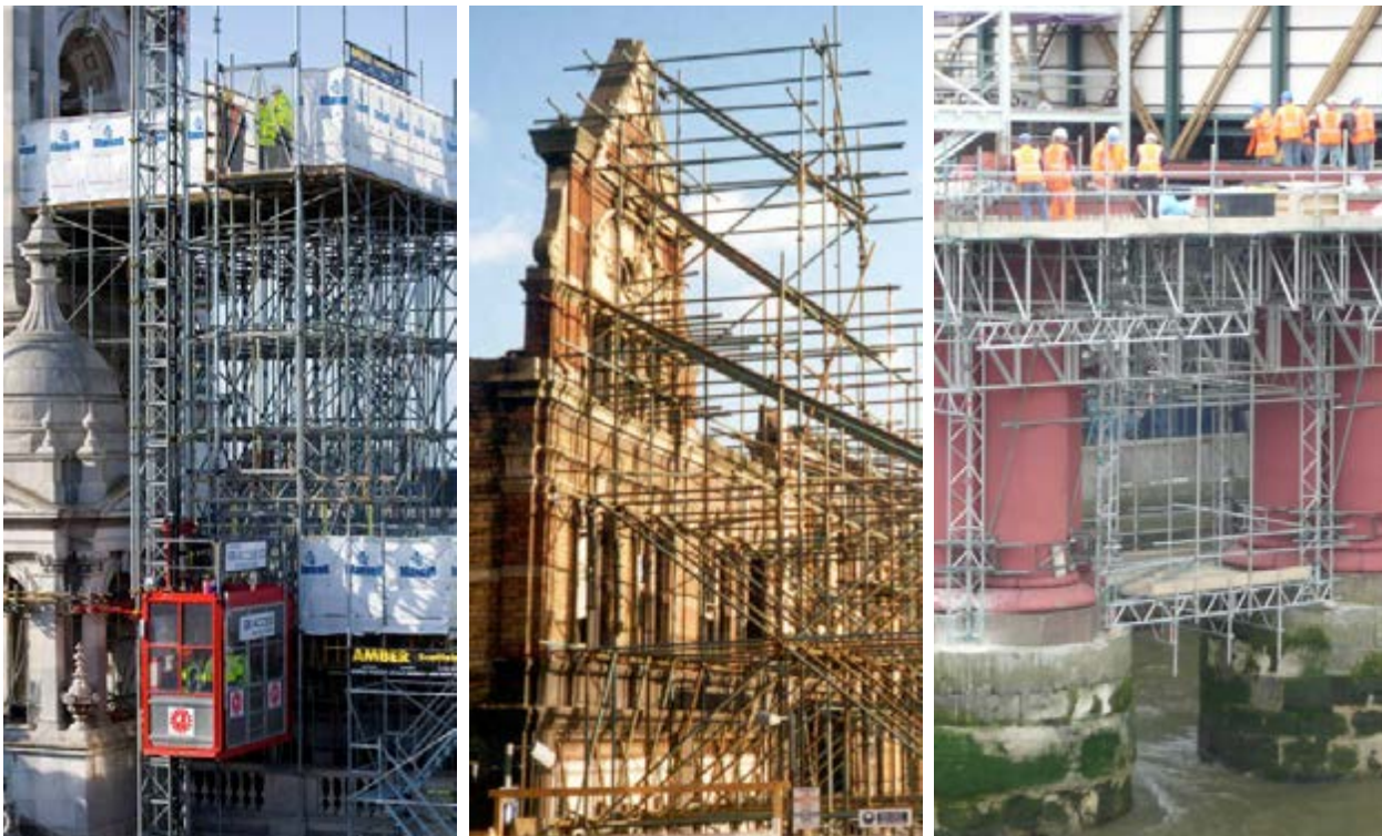
Fig 2. Examples of scaffold structures that would require bespoke design and significant procedural control
