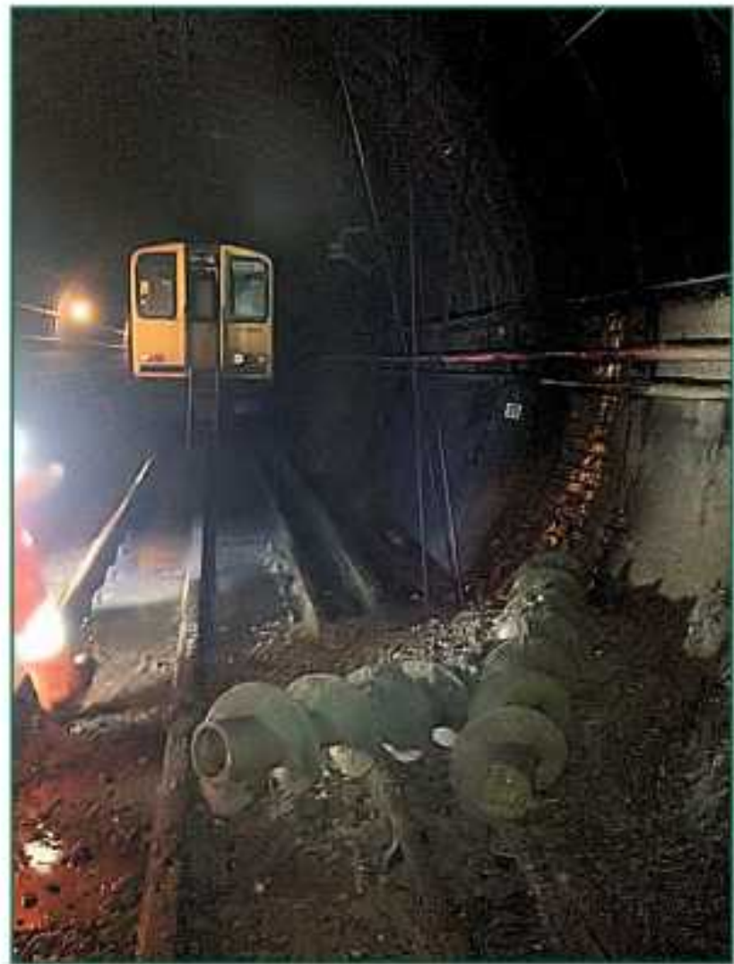
Figure 6: Auger sections and debris on the track (photograph courtesy of Network Rail)
