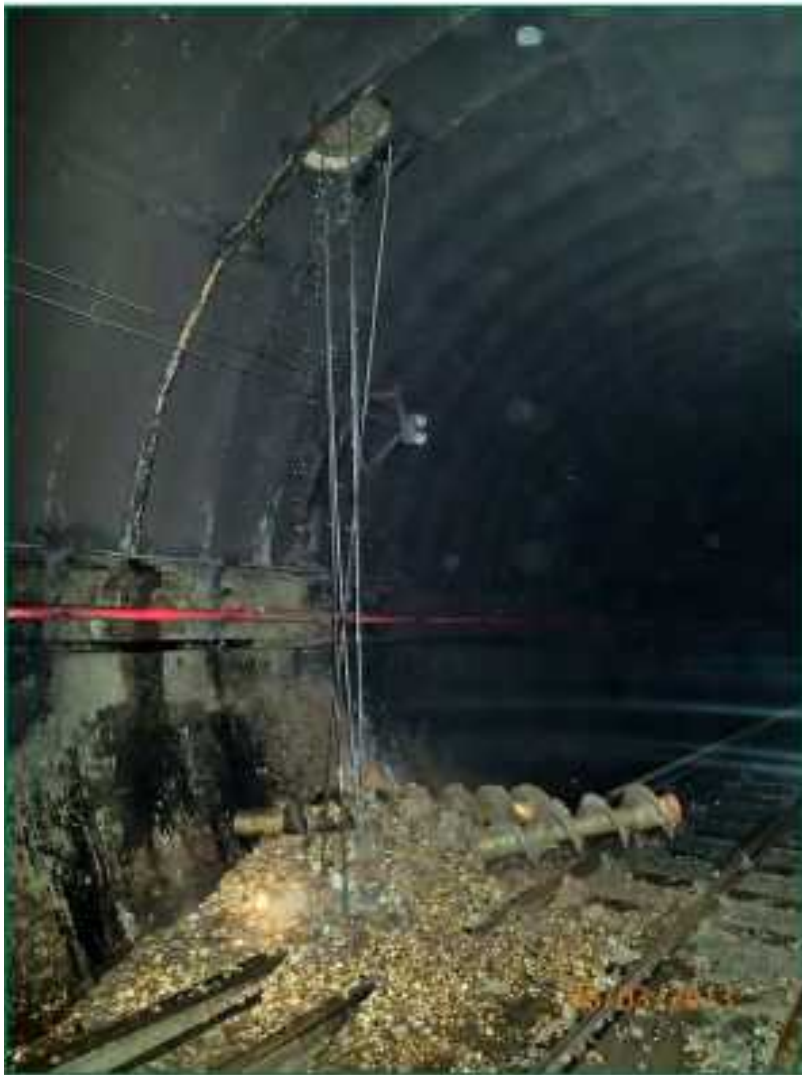
Figure 5: Penetration of tunnel lining and debris on track
